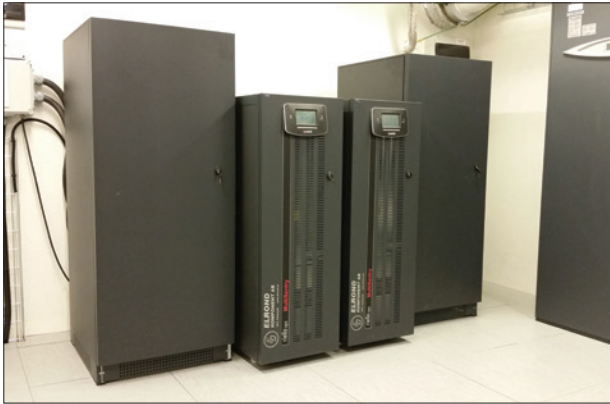
Datahall 2x40kVA parallell
