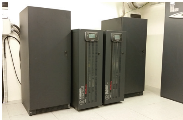
Datahall 2x40kVA parallell
