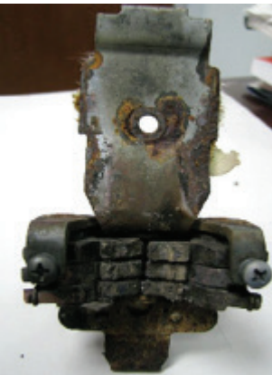
Fig 28: Circuit breaker corrosion
